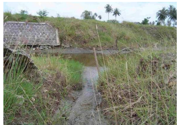
Figure 3 Drainage Entering Main Channel
